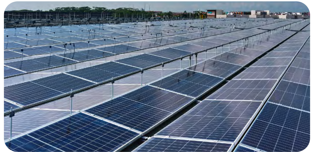
| STT GDC's rooftop solar photovoltaic system in Loyang
